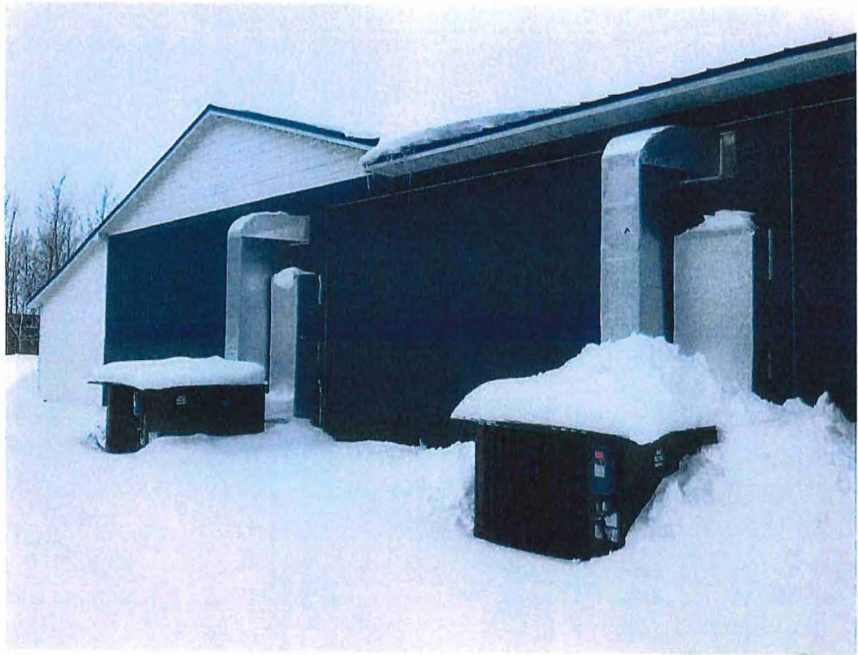
Canopy and HVAC southwest
