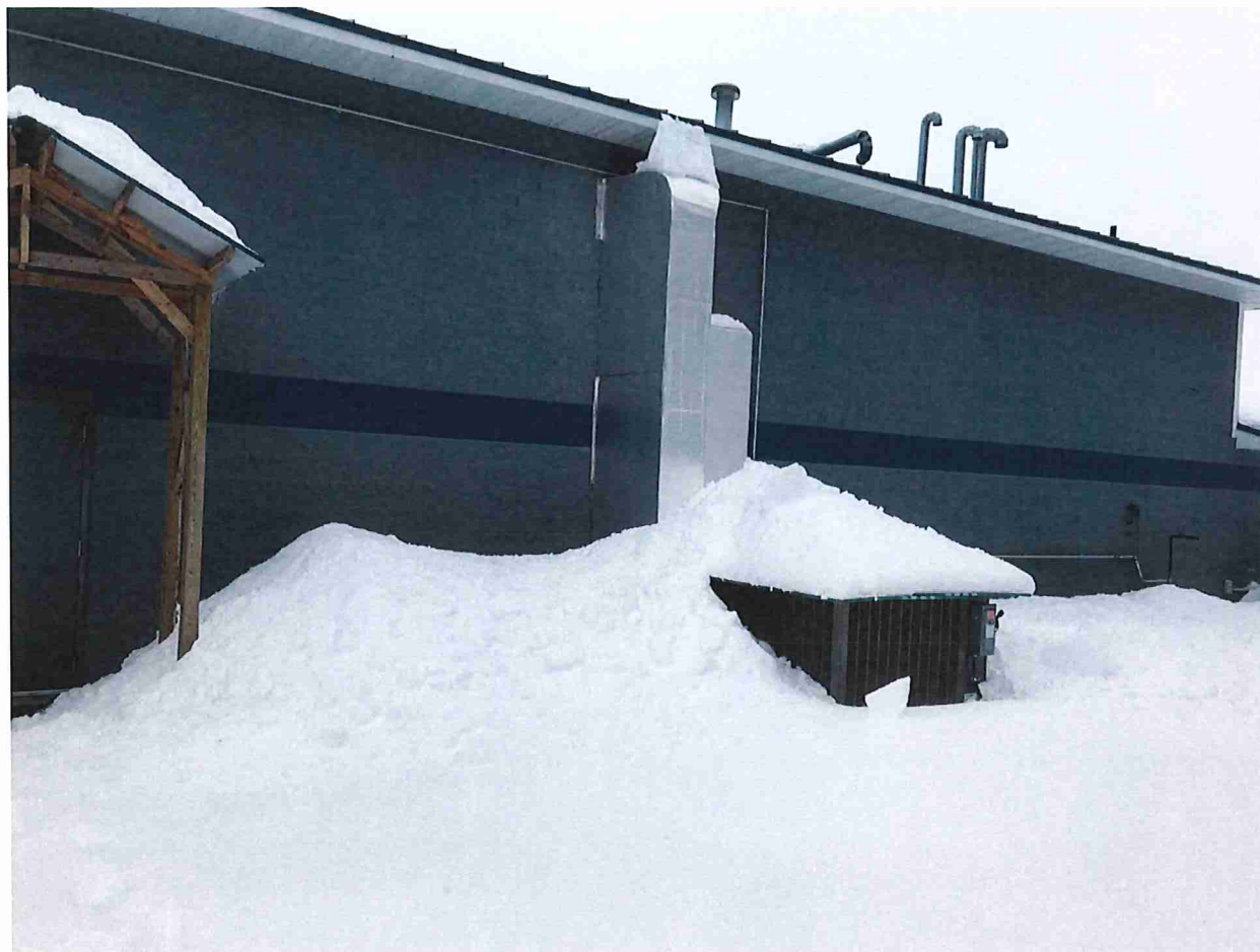
Canopy and HVAC southeast
