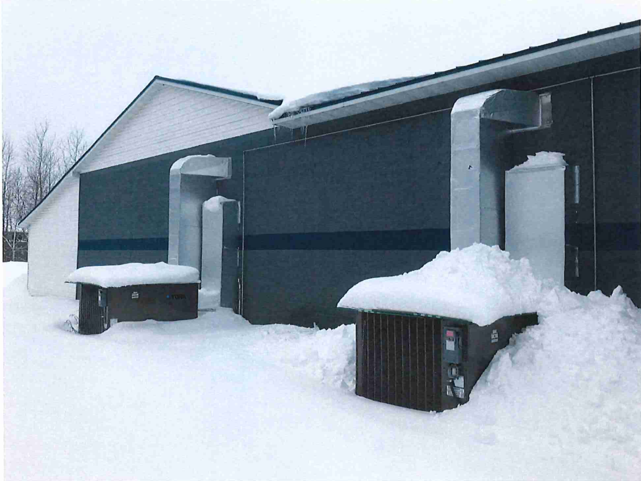
Canopy and HVAC southwest
