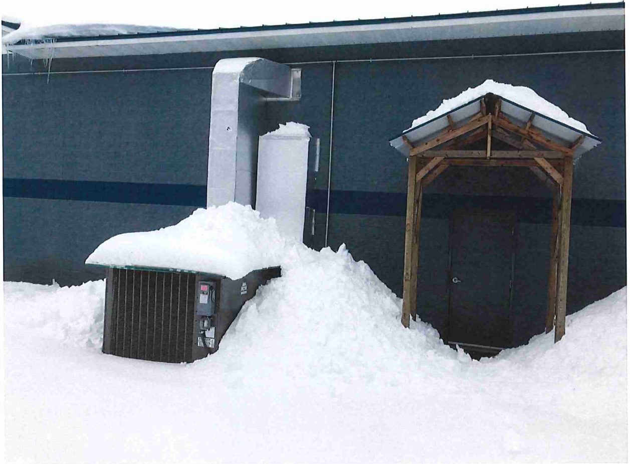
Canopy and HVAC south middle
